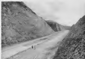
A big problem faced by the highway engineers was the enormous amount of earth that had to be moved. This view shows large excavations that made possible a highway which will reduce present travel time by 45 minutes.
